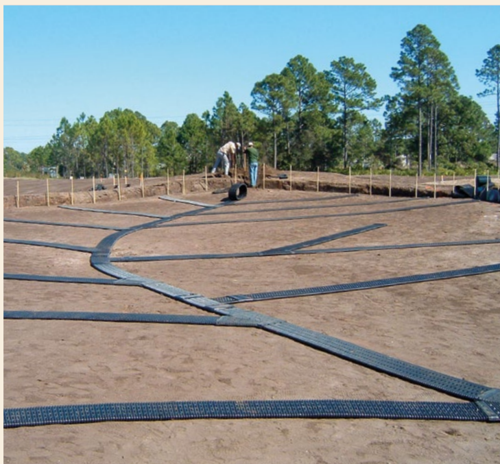
The AdvanEdge solution can be used by clubs to improve subsurface drainage on their golf courses
